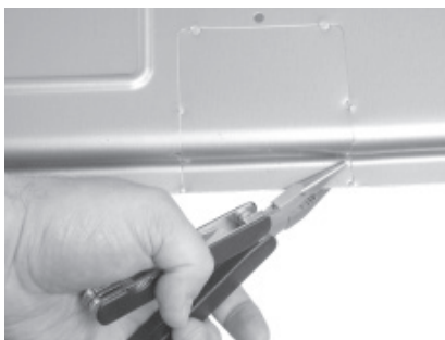
FIGURE 11 REMOVING CONDENSATE KNOCKOUT
